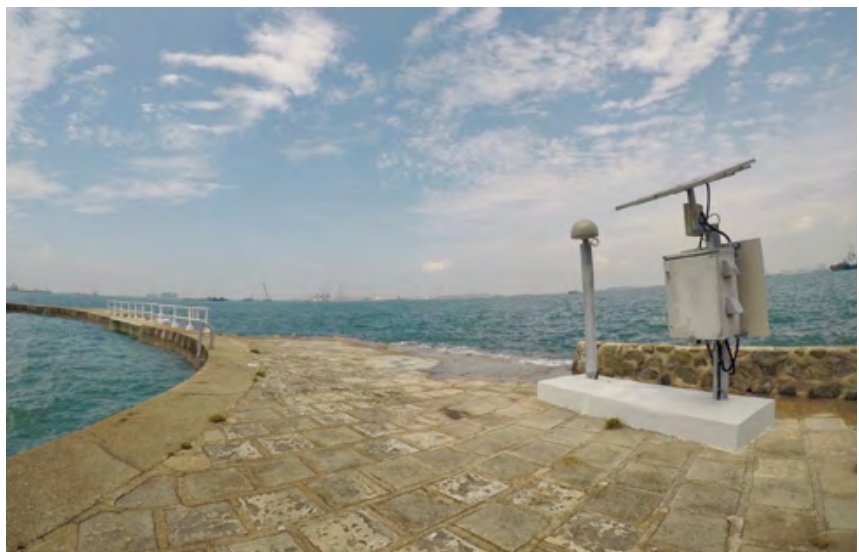
The GNSS Reference Station on Sultan Shoal (SSTS). Image: Singapore Land Authority (SLA).
