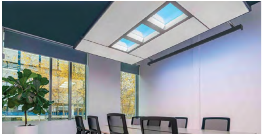
Circadian lighting installation on the ground floor of the Signify offices in Eindhoven, Netherlands. Circadian lighting supports and enhances the productivity of employees.
